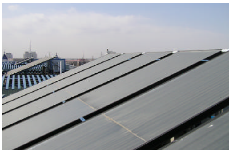
Figure 8 Solar water heating system on roof in China
